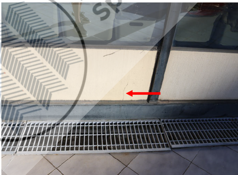
Fine cracking in the north wall on the level 3 balcony, east side.
