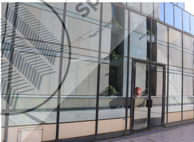
North wall on the level 3 balcony, west side.
