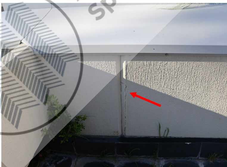
Slight cracking in the south boundary wall on the level 3 balcony, east side.
