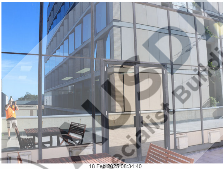
North wall on the level 3 balcony, west side.
